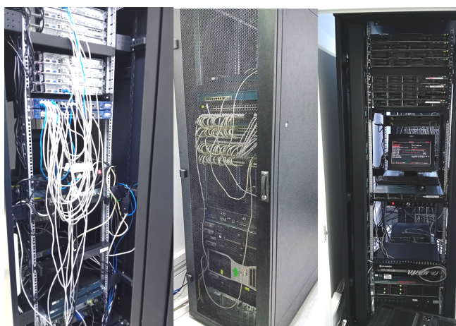
Fig.1. 10 Node NBU Micro Cloud Installed
